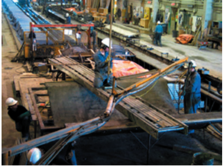
2. A uniform thickness of Glass fiber Reinforced Concrete (GFRC) is applied to the hanging fabric.
