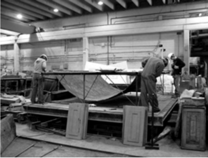
1. A flat rectangular sheet of geotextile fabric is hung from a steel frame
