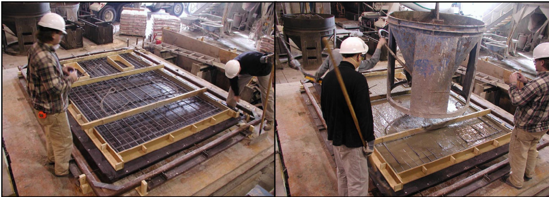
Figure 9. securing fabric, placing reinforcement and concrete in full-scale wall panel formwork (C.A.S.T. photos).
