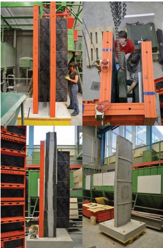
Figure 18: Demonstrator: Mechanical Wax Properties and Handling - Assembly and casting of a 3m high concrete column on wax formwork with a steel support structure.
